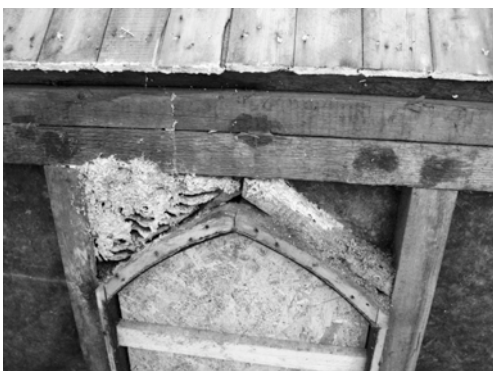
Figure 10. St Fillan's Episcopal Church: arched window construction exposed during the repair works (2011). Note, a perfect place for wasps!
