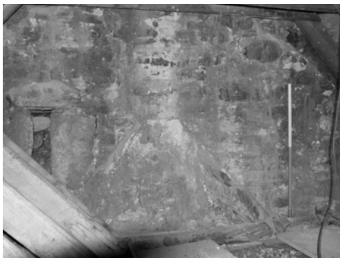
Figure 8. Evidence in the form of a raggle line on the west gable end of 42–44 High Street, preserved in the roof space of numbers 38–42. (© National Trust for Scotland)
