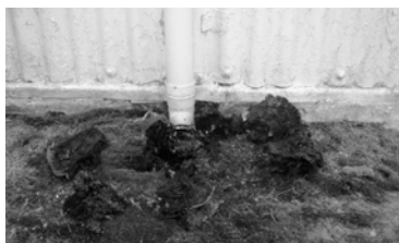
Figure 12. Build-up of ground vegetation due to inadequate removal of rainwater (2009).
