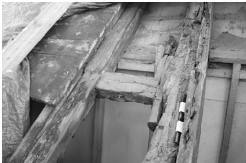
Figure 6. One of the bridle beams fixed to both the east and west pitch of the south roof. (© National Trust for Scotland)
