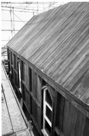
Figure 13. St Fillan's Episcopal Church: the corrugated-iron sheeting removed, the timber shell of the building is revealed (2011).
